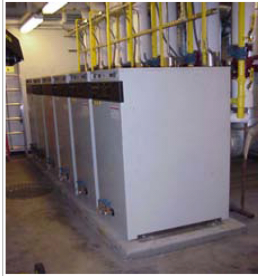
Figure 6.02 LBNL replaced two boilers with 11 modular boilers to maximize part-load efficiency. (Source: LBNL)
